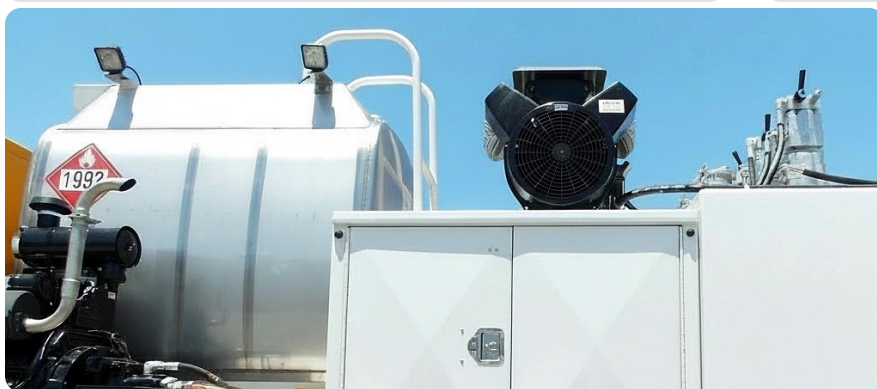
Compressor, hydraulic power unit & pumps.
