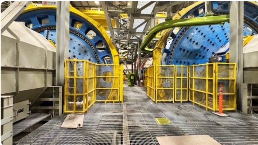
Twin monorail rails spanning the walkway between grinding mills.
